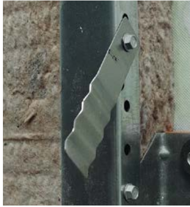
Stainless steel strap mechanically attached to the side of rain screen girt and then bent in place to secure mineral wool insulation.
