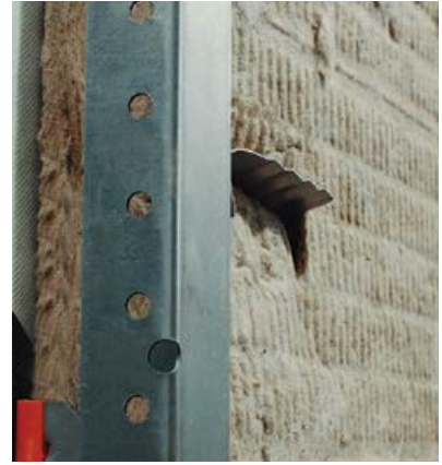
Thermally efficient method for rain screen attachment and mineral wool insulation. Note the red bushings that thermally isolate the vertical girts.
